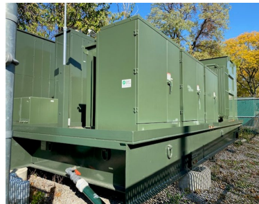
Acoustic Sensing at Medium-voltage Transformer
